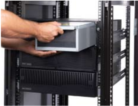
Hot swappable batteries
